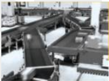
Good Conveyor Management
